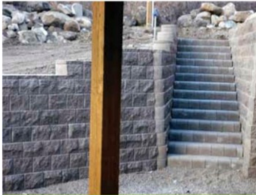
There are many ways to tackle features and stairs with terraforce. It has been stated that: "Working with these blocks is like therapy."
